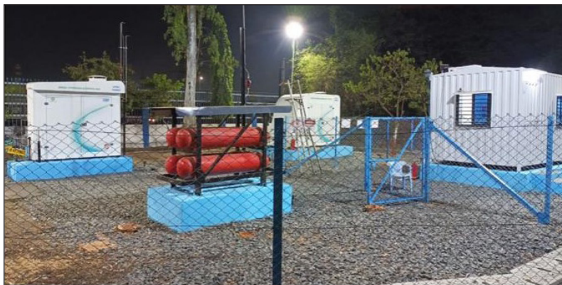
Figure 2: Project view at NTPC Kawas
